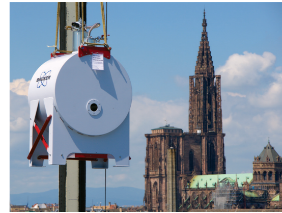
Weighing approximately two tons, the Solarix FTMS was installed via the roof of the IBMP. © Jean-Luc Evrard
